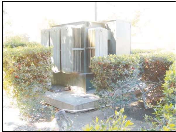
Electrical transformer in north central portion of subject property
